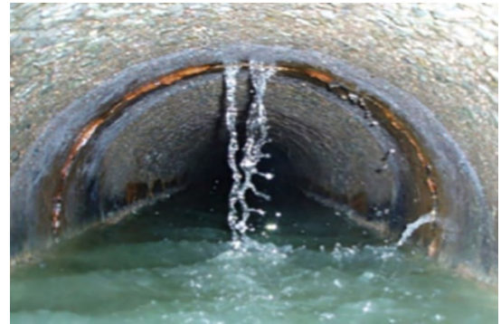
FIGURE 3. Example of Sanitary Sewer Infiltration
