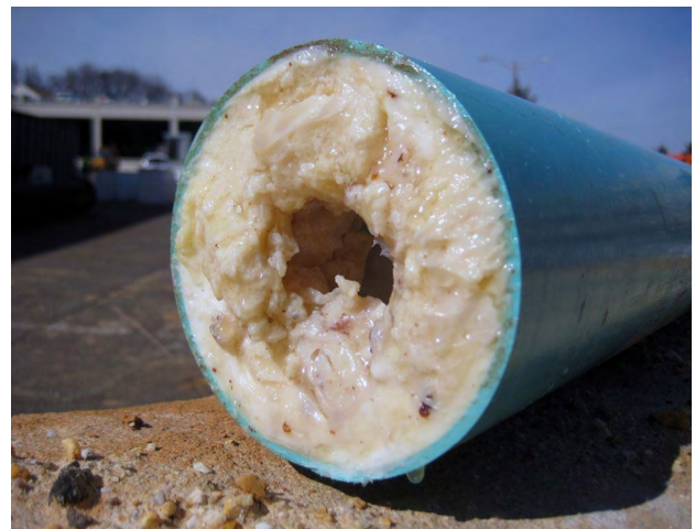
FIGURE 7. FOG buildup in PVC pipe in Huntsville, TX
